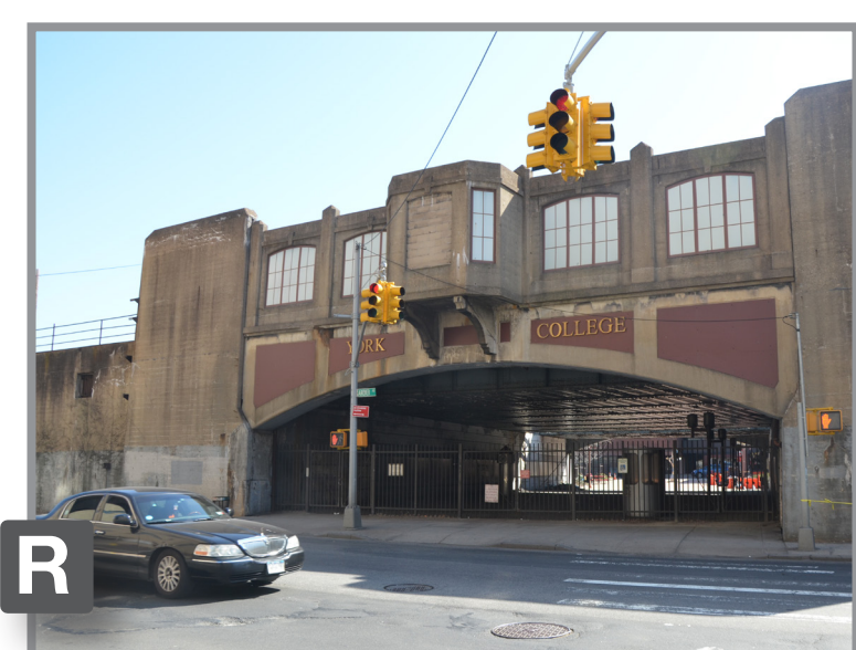
R Strong desire lines to York College. Viaduct is a barrier for pedestrian movement and tunnel conditions are poor.
