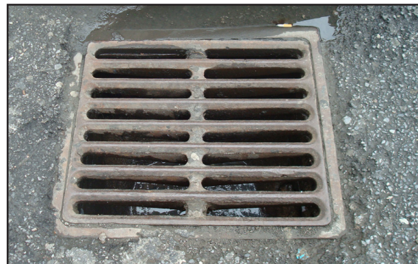
Drainage grate with large openings are unsafe for cyclists
