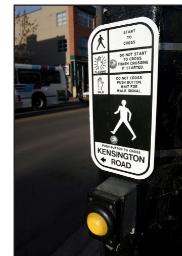
Pedestrian actuated signal, Calgary, Canada, Photo: PBIC
