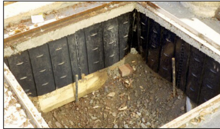
Root barriers prevent the roots from lifting the sidewalk but curtail growth
