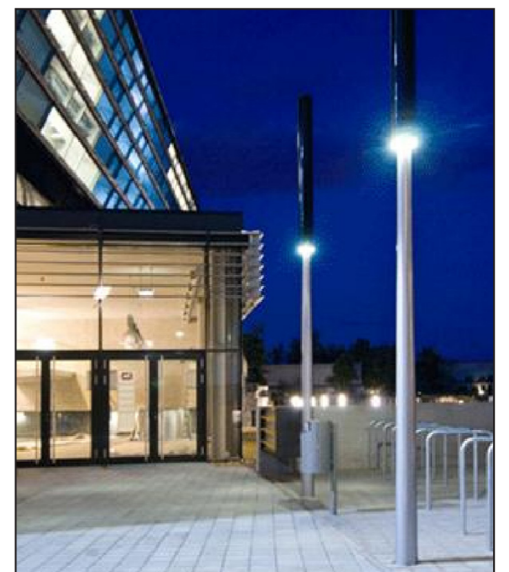
Solar powered LED plaza lighting, Spain
