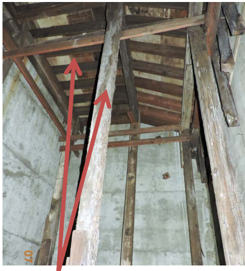
Formwork left in place
