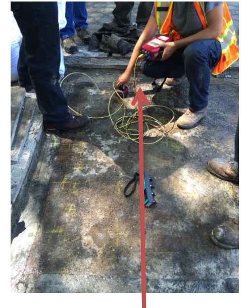
Linear Polarization Resistance to obtain corrosion rates
