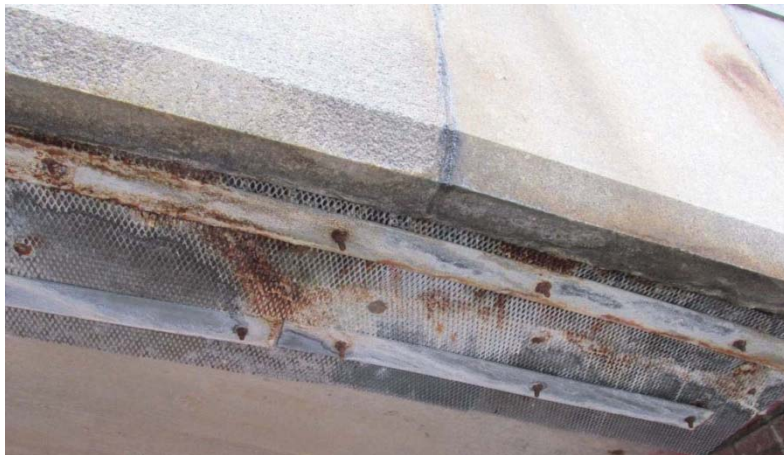
Wire Mesh Corrosion from Leakage
